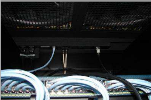
Containment Cooling system view looking inside rear door
